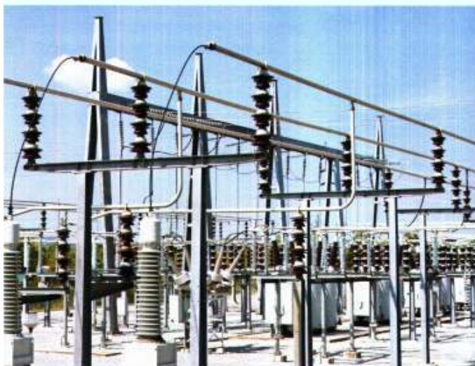
Electricity Power Station
