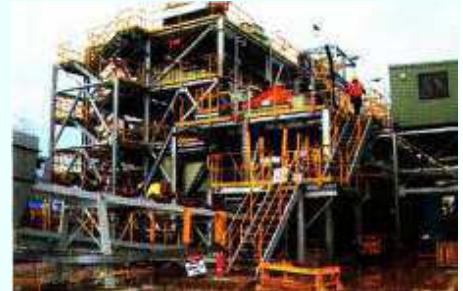
Part of the efficient operation
